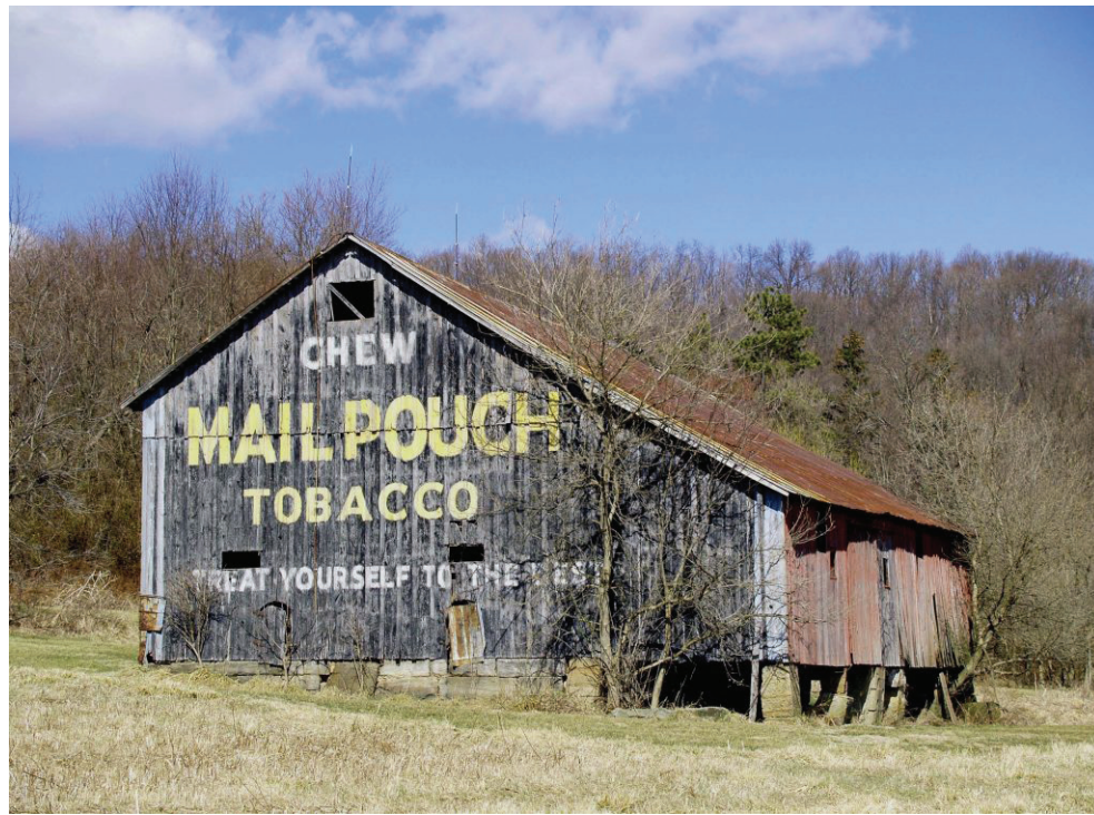
Above: The wood may be deteriorating and the paint may be fading, but this Mail Pouch barn near Newark, Ohio, still stands.
