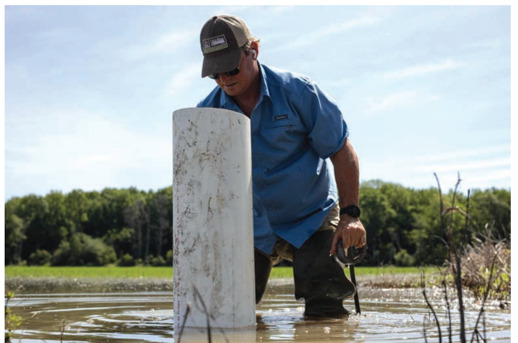
Above: Blake Gerard looks down a pipe he installed in a rice field. The pipe, known as a riser, helps control the water level in his rice field. (Lylee Gibbs photo)
